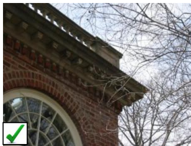
Decorative moldings and cornice lines on buildings with flat roof lines add visual interest.
